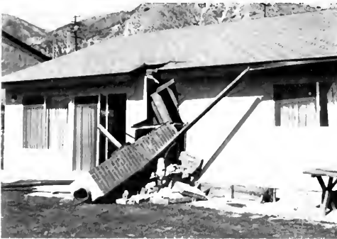
Photo 25. Collapse of chimneys was the most prominent damage to residential structures. Courtesy of Charles A. Yelverton.
